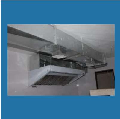
Commercial Kitchen Chimney
