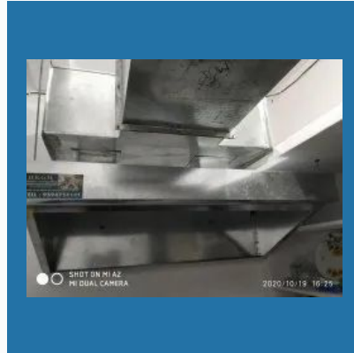
Exhaust Ducting And Air Fresh
