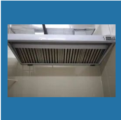
Kitchen Exhaust System
